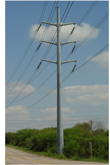
Solid Pole Structure
